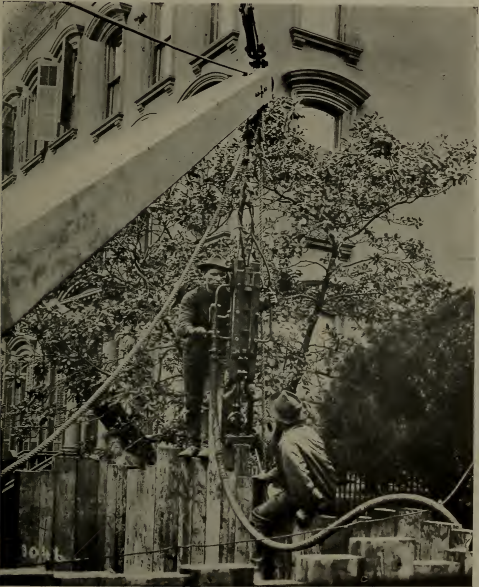
Driving Sheet Piling with an Ingersoll-Rand Sheet Pile Driver on Subway Construction in Brooklyn.
